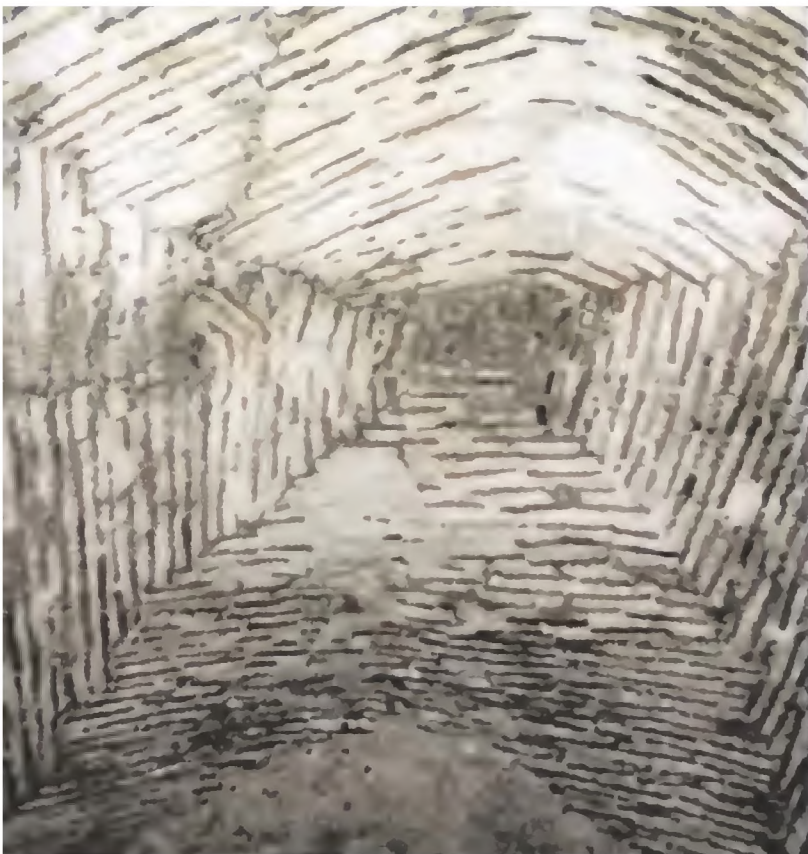
• View of the ceiling of Virgin Mary Church, It is covered with the tiles crossshaped
